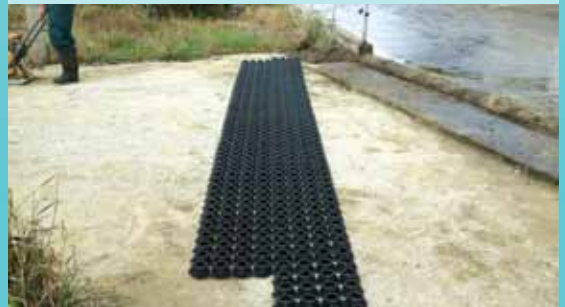
4. Start laying SurePave Panels from left to right ensuring they interlock together correctly
